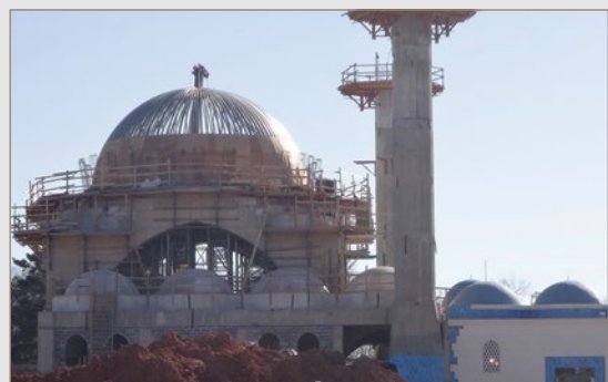
Photos: Turkish American Community Center, MD Images courtesy of Fachina Construction Company
